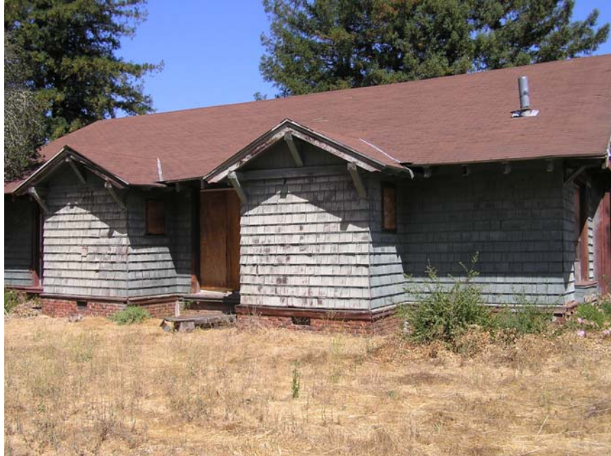
Image 5. Alma College Chapel, existing exterior view of the south facade. As the most exposed side of the building, the wood deterioration is more severe than other sides. (Knapp Architects, digital photograph, 2009)
