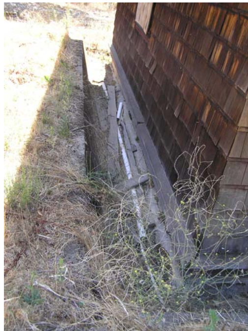
Image 39. Alma College Classroom Building, existing exterior view of retaining wall at east façade which creates a partial moat where vegetation and debris have collected. (Knapp Architects, digital photograph, 2009)
