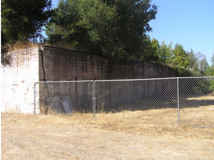
Image 60. Alma College Tevis House / Faculty Residence ruin, exterior view looking northwest at the retaining wall that supported a west portion of the house. A large crack in the concrete retaining wall is seen at the left near the wall corner. (Knapp Architects, digital photograph, 2009)
