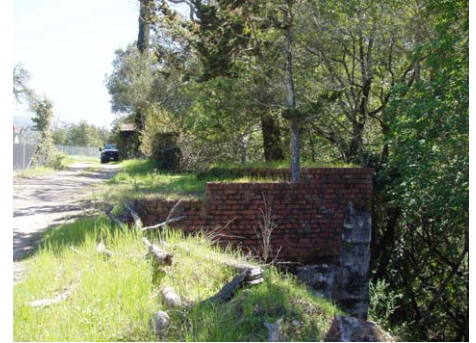
Item 12 0904xx Brick retaining wall on
