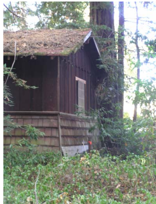
Image 68. Alma College Wood Shed, existing exterior view of south façade (left) east façade (right). The roof and walls are partially collapsed. Vegetation debris has collected on the roof. (Knapp Architects, digital photograph, 2009)
