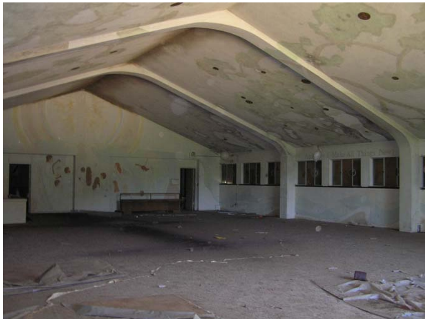
Image 25. Alma College 1949 Library addition, existing interior view looking east. Murals at the ceiling and walls are visible. A band of windows is seen at the right. Brown staining at the peak of the vault implies water infiltration. (Knapp Architects, digital photograph, 2009)
