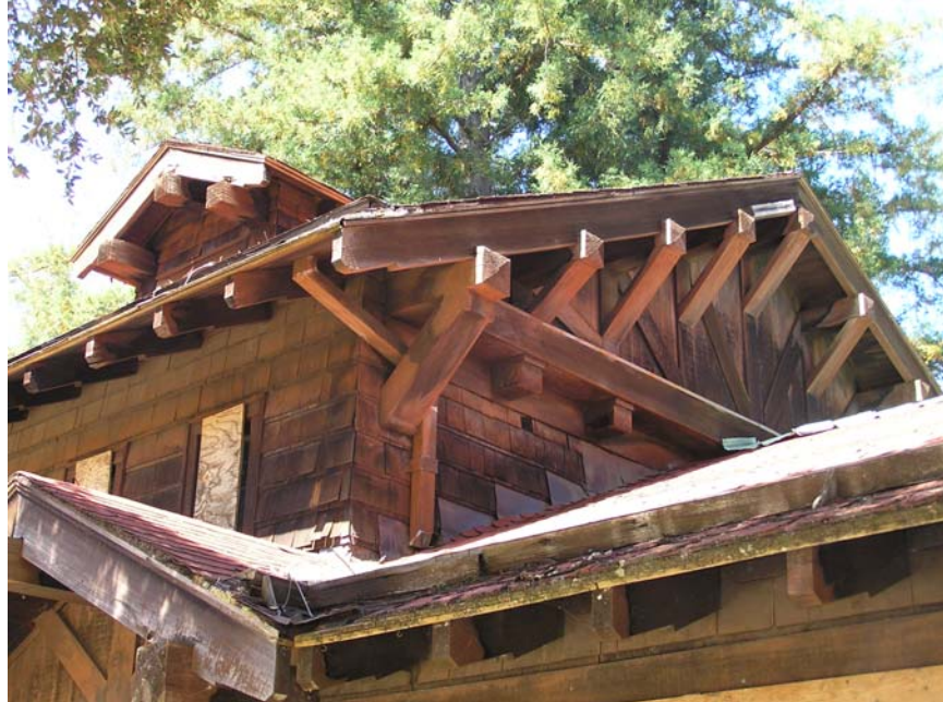
Image 17. Alma College 1934 Library, existing lower east roof, upper roof and roof dormer viewed from the southeast. The woodwork, roof material and sheathing are deteriorated. (Knapp Architects, digital photograph, 2009)
