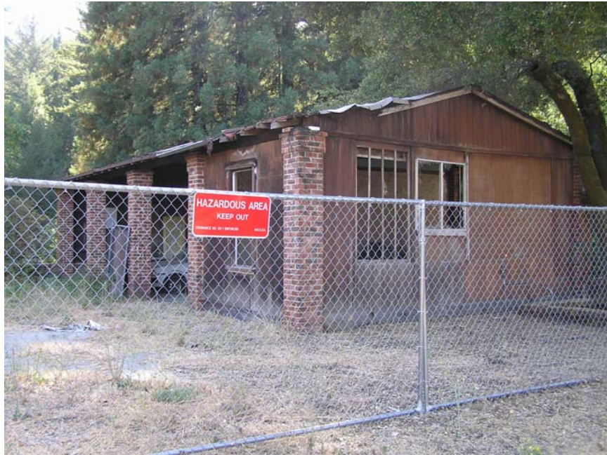
Image 65. Alma College Garage/Residence, existing exterior view from the northeast. The brick piers at the four carport openings are shown with wood infill. (Knapp Architects, digital photograph, 2009)
