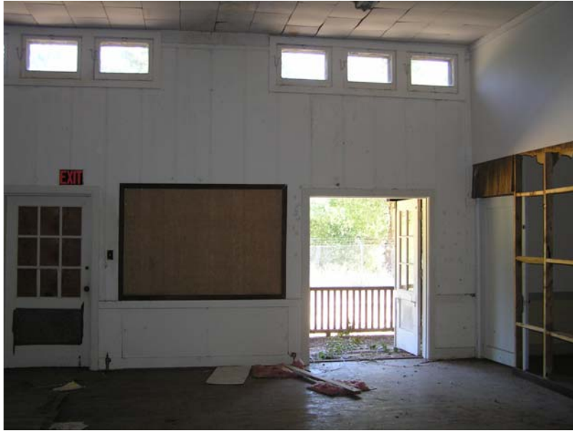
Image 40. Alma College Classroom Building, existing interior view looking north at a classroom entry to the exterior arcade and upper clerestory windows. Historic wood paneling and trimwork is intact. The finish at the partition wall at the right is partially removed. (Knapp Architects, digital photograph, 2009)
