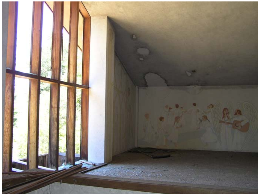
Image 28. Alma College 1949 Library, existing interior view of full-height west window and mural at north wall. The west window framing is substantially intact but the glazing is broken. (Knapp Architects, digital photograph, 2009)
