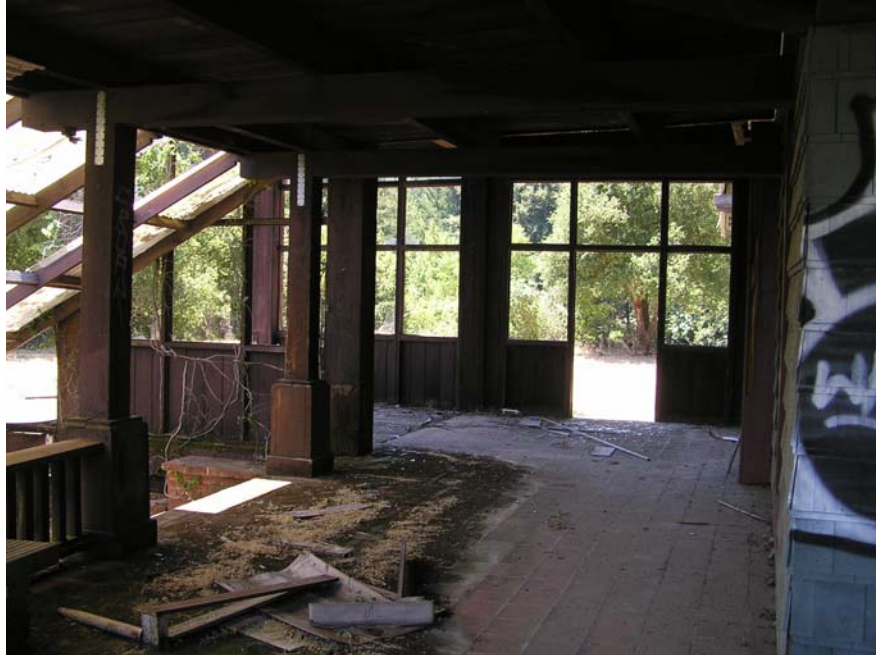
Image 48. Alma College East Walkway beyond, existing view inside the North Walkway from the northeast corner of the Chapel. At the left, a brick stair, covered by a shed roof with corrugated plastic, leads to the Chapel basement entry . Vegetation growth is seen at the veranda clay tile. (Knapp Architects, digital
