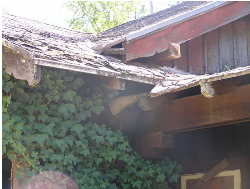
Image 38. Alma College Classroom Building, existing exterior view of roofline at main south entry porch at left. The roofing and wood sheathing are deteriorated. Vegetation growth on the building brings moisture that increases wood deterioration. (Knapp Architects, digital photograph, 2009)
