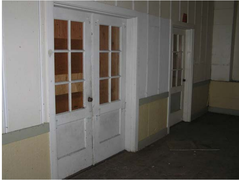
Image 42. Alma College Classroom Building, existing interior view of original intact glazed doors. (Knapp Architects, digital photograph, 2009)
