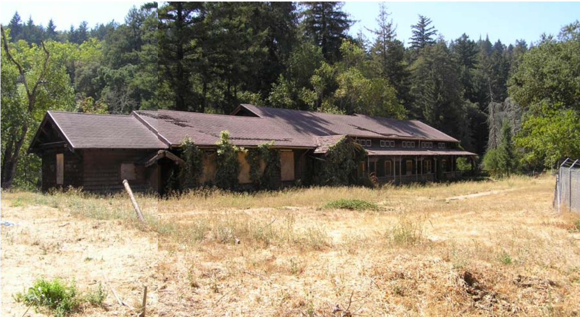
Image 31. Alma College Classroom Building, existing exterior view of north façade. The dark lines at the roof are displacement cracks where the roof form is warped ((Knapp Architects, digital photograph, 2009)
